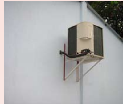
Our Rotary grant enabled the school to install this new air conditioning unit
