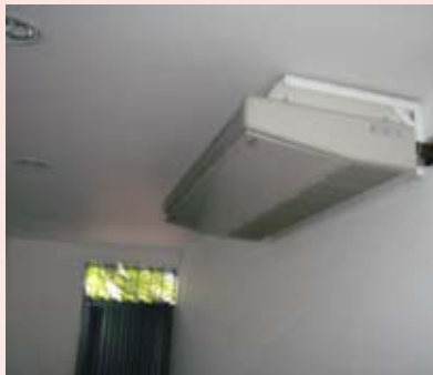
Air conditioning unit inside the computer lab
